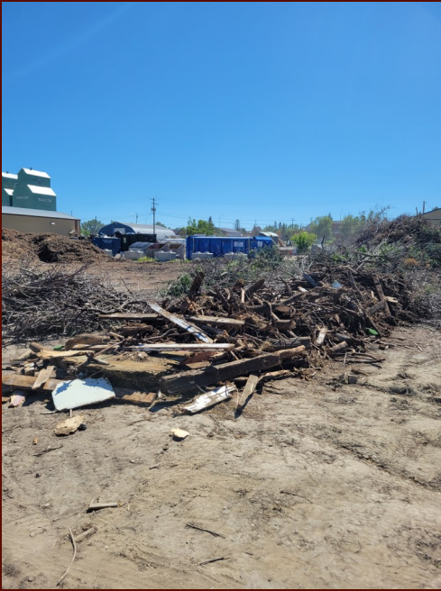
Illegal construction waste dumping in yard waste areas.
